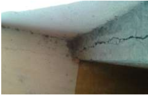
Fig.1 Crack on beam
